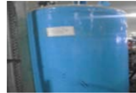
Air reservoir tank
