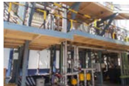
Installed new set up for deaerators at Chopanki site to use HI curing line dome flash steam.
