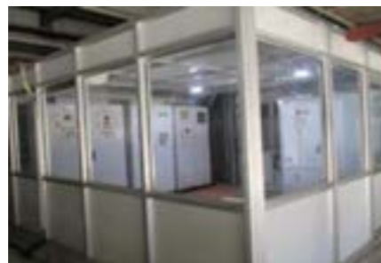
Installed live VFO panels in the utility section to replace Star-Delta starters, using PIO controllers for motor RPM control.
